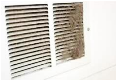
NO DIRTY VENTS
