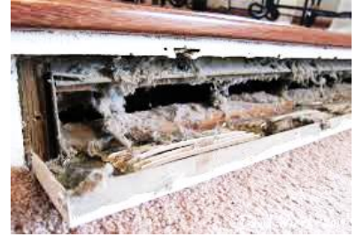
NO DIRTY DUCTS
